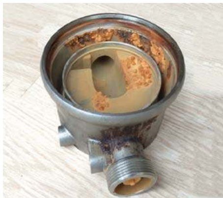
Figure 1: The foot of a pump constructed in stainless steel AISI 304 affected by MIC (photo: Innomet private company)
